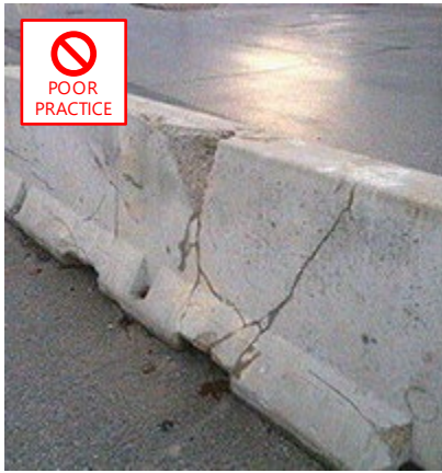
Figure 10. Structurally deficient barrier. Source: John Shaw
