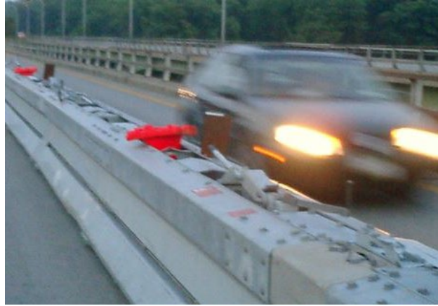
Figure 39. Steel barrier system in a bridge application.
