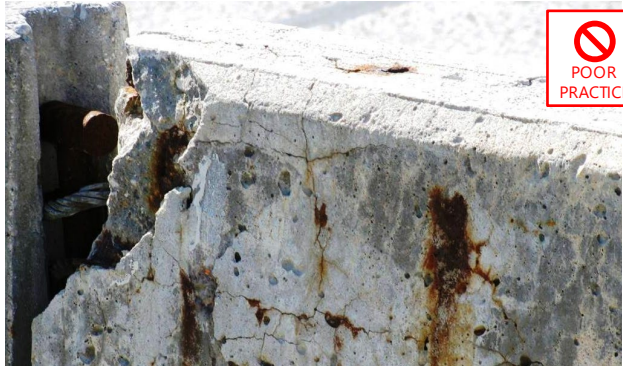
Figure 32. Structurally deficient barrier: spalling concrete. Source: Wisconsin DOT
