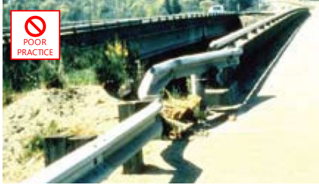
Figure 13. Pocketing of a permanent steel beam guard adjacent to a rigid bridge parapet.
