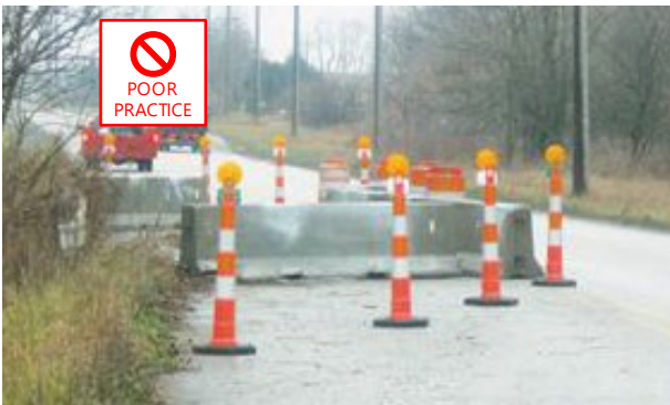
Figure 16. Barriers incorrectly used to screen off an excavation. Source: Wisconsin DOT
