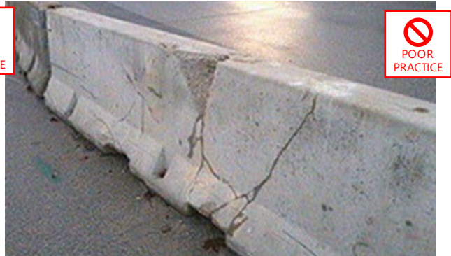
Figure 33. Physically damaged concrete barrier. Source: John Shaw
