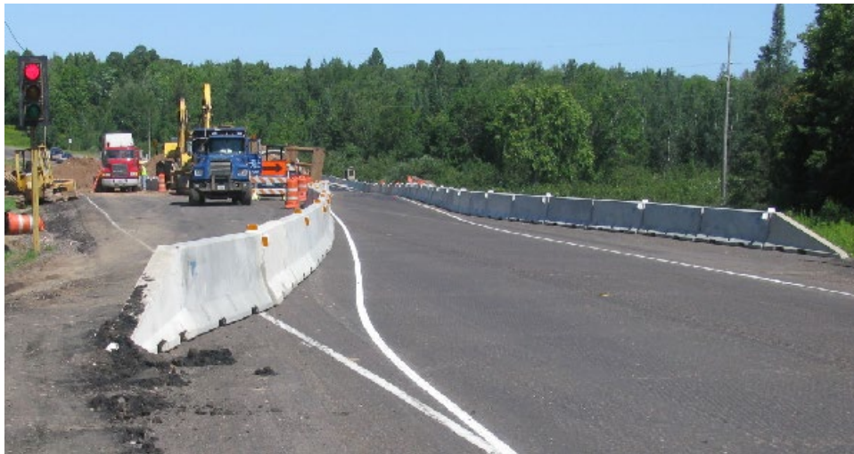
Figure 26. Flared temporary portable concrete barrier system terminated outside of clear zone.
