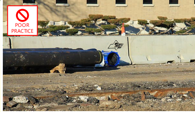
Figure 14. Construction materials stockpiled next to barriers can alter vehicle deflections.
