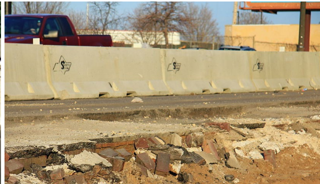
Figure 2. Barrier can provide protection against edge drops. Source: Wikimedia Commons/Michael Hicks
