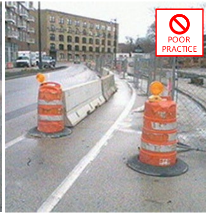
Figure 11. Barrier incorrectly used without crashworthy end treatment. Source: John Shaw
