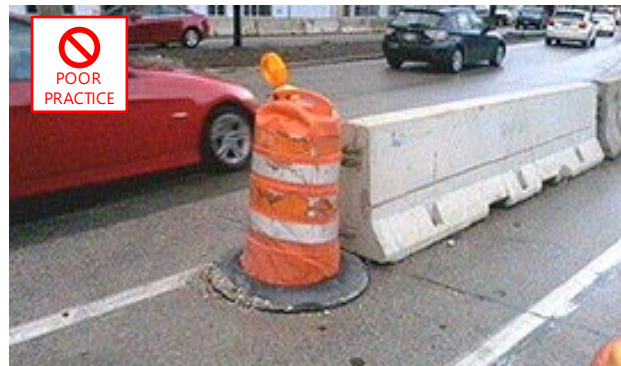
Figure 17. Barrier incorrectly used without crashworthy end treatment. Source: John Shaw
