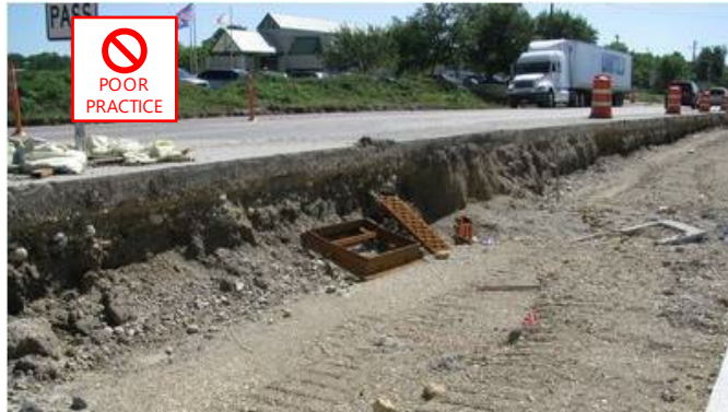
Figure 65. Abrupt pavement edge drops creates the potential for serious crashes.
