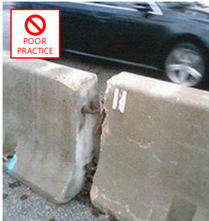
Figure 9. Barrier with missing and bent connectors. Source: John Shaw
